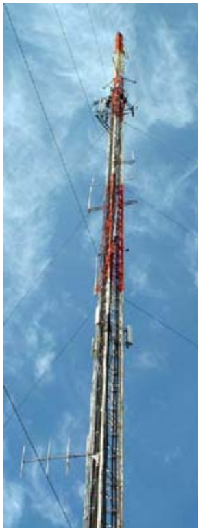
Repeater site tower. The Diamond dual-band antenna for 2 meters is visible on the left side, above three new panel antennas for Sprint. The 440 antenna is on the left, above 2 meters.
