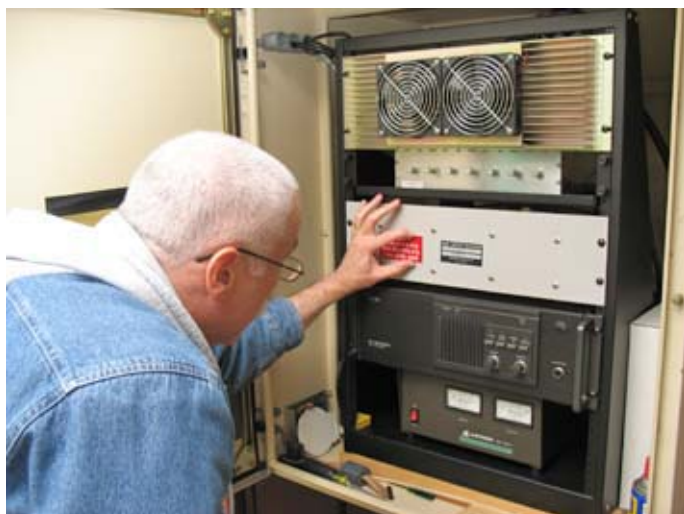
Greg, KB2CQE adds a new label to the 449.925 MHz repeater on a recent maintenance visit to the site.
