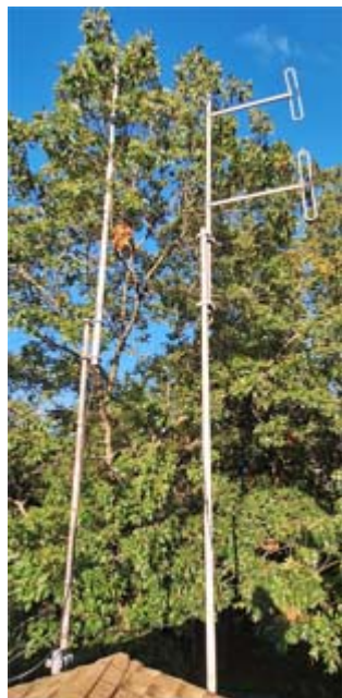
440 antenna (left) and Sinclair exposed dipoles for 2 meters (right) after work by Bob N2CBH and Lou KD2ITZ. [KD2ITZ pic.]
