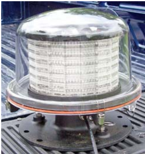
Aircraft warning beacon for the Empire State Building as replaced last summer.
