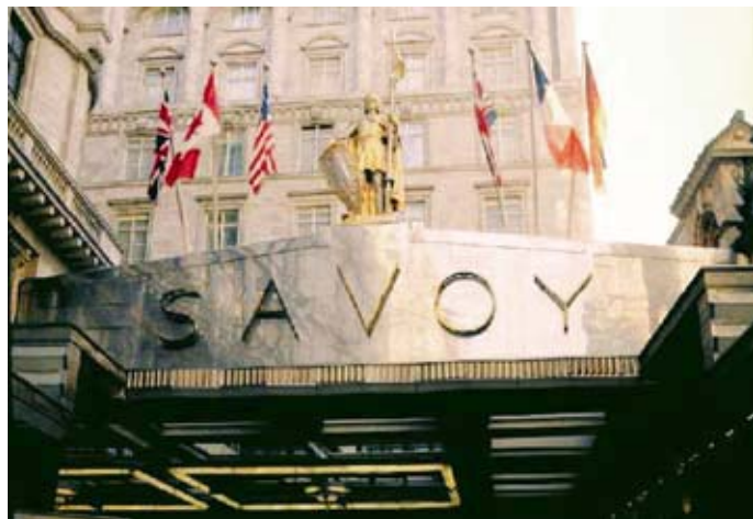
The 70-year old stainless steel entrance canopy to London's Savoy Hotel was cleaned, repaired and reinstalled in 1999.
